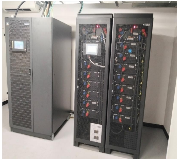
Figure 2. UPS and Li-ion battery setup during operation
