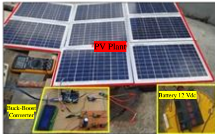
Fig. 11. PV generator systems
