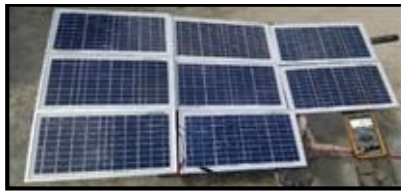
Fig. 5 Photovoltaic Power Plant
