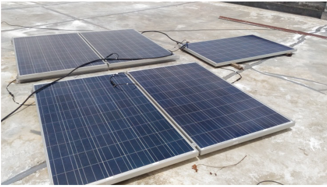
Fig 5. Rooftop PV Installation Capacity 1.25 kWp
