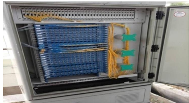
Figure 4: Optical Distribution Cabinet
